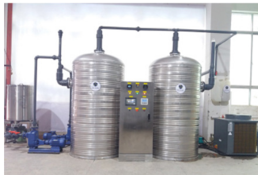
Figure 11. The visual aspect of automated biodigester
